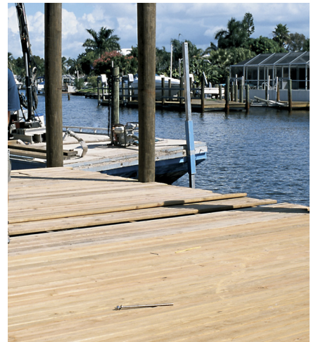
Elevated Service / Severe
